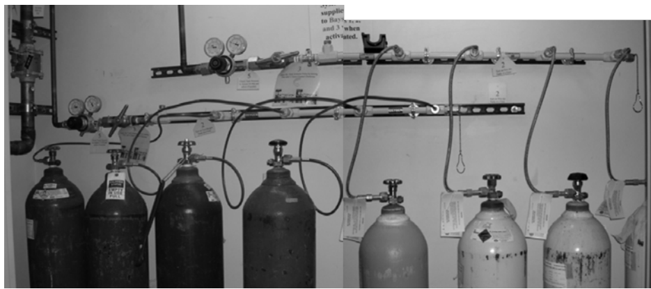
Figure 2: Existing reserve cylinder room at UIHC
