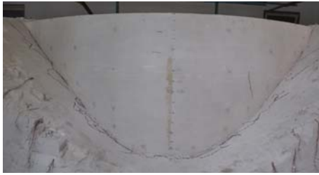
FIGURE 20: The final distribution of upstream cracks.
