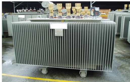
Gambar 2.6 Transformator (Sumber: PT. XYZ)
