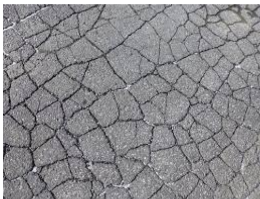
Gambar 2.2. Alligator Cracking (Pramestya, 2018).
